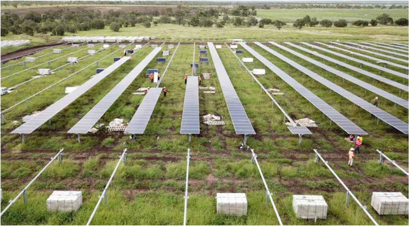
Whitsunday Solar Farm. Image Courtesy: Edify Energy
